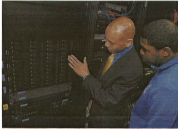
Photo submitted by John Oates/SU Office of Public Affairs IBM executive Elmer Corbin, left, explains an IBM BladeCenter to Claudis Gein, a Southern University senior electrical engineering student from Mansura. The IBM equipment will help Southern create a cloud-computing platform for consolidating its servers.
